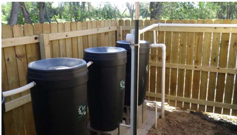
Plumbing of roof and rain gutters connecting to the rainwater harvesting collection system, northeast corner of bathroom looking to the southeast.
