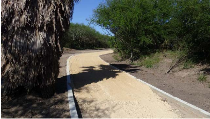
Heading west/northwest. Subgrade is being added and compacted to form the base of the trail.
