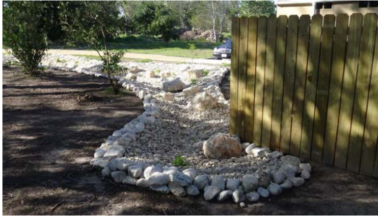
Swale adjacent to privacy fence to protect rainwater harvesting system behind bathrooms.
