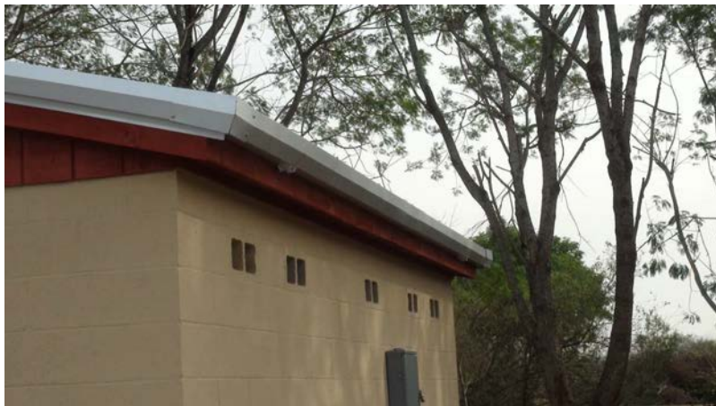
Rain gutters have already installed to capture and divert rainwater into the rain harvesting cistern and rain garden. The holes in the gutters for the downspouts have already been cut out.
