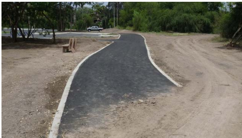
The trail leading up to the parking lot. The contractor has placed dirt over the trail to use as a road for their equipment. The dirt will protect the trail from being damaged the vehicle traffic going over it.
