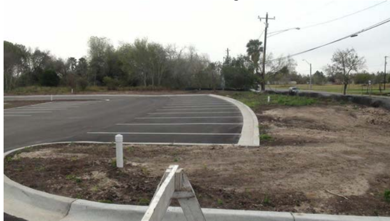
Entering the parking lot looking to the S-SE. Note the curved design of the parking lot. Curves and irregular shapes are utilized throughout the parking lot and bio-retention basin.
