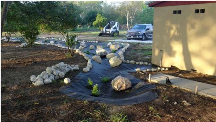
NE end of swale looking to the SW from behind the bathroom. Pad for cistern shows proximity of cistern to the swale.
