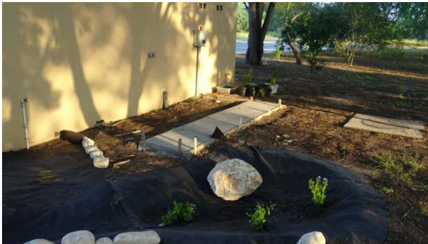
Concrete pad behind bathrooms to be used as the base to support the rainwater harvesting cistern.
