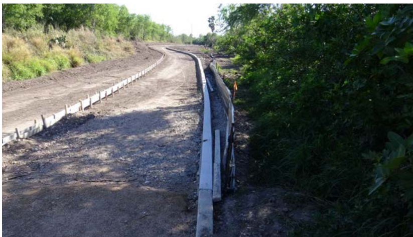
Heading north/northeast, the forms and curb are visible. The grade of the walking trail has also been reached and is ready to receive the sub-grade material.
