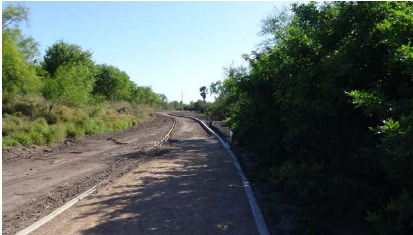
The concrete form is visible on the left side of the photo and the completed concrete curb is visible on the right.
