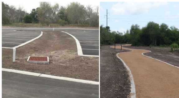
The City of Los Fresnos installed LID elements at the nature park, including a bio-retention basin in the parking lot. Other LID elements include bioswales, pervious walking trails and a rainwater collection system.
