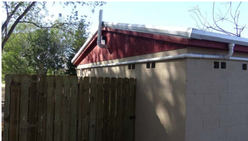
Plumbing of roof and rain gutters connecting to the rainwater harvesting collection system, northeast corner of bathroom looking southwest.
