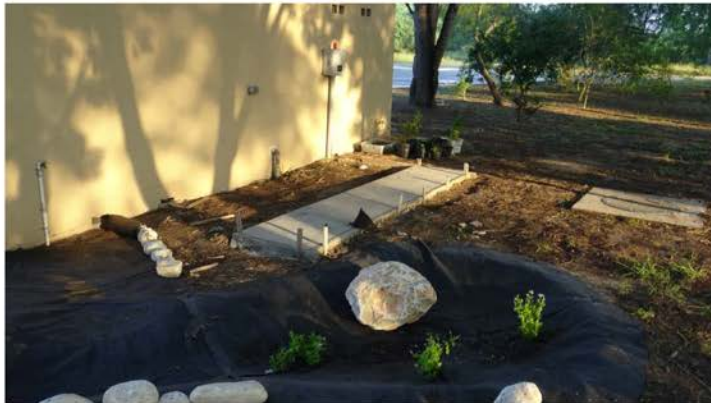
Concrete pad behind bathrooms to be used as the base to support the rainwater harvesting cistern.
