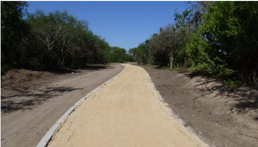
Heading west. The high school is to the north of the trail. Subgrade for the trail has already been compacted in this portion of the trail.
