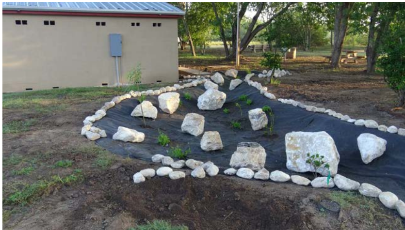
Vegetative swale and rain garden being installed and connected to the rainwater harvesting cistern to be installed behind the public restrooms.
