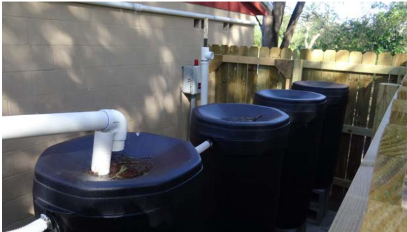
Southeast end of privacy fence looking at the rainwater harvesting collection system behind the bathrooms looking to the northwest.
