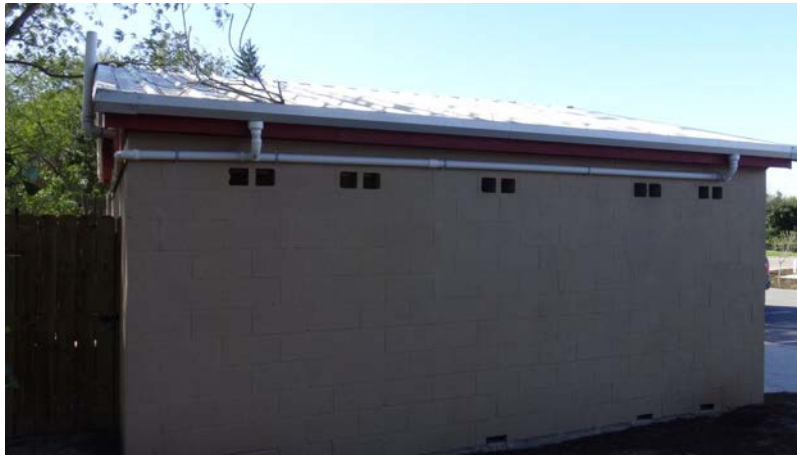
Plumbing of roof and rain gutters connecting to the rainwater harvesting collection system, north end of bathrooms looking south.
