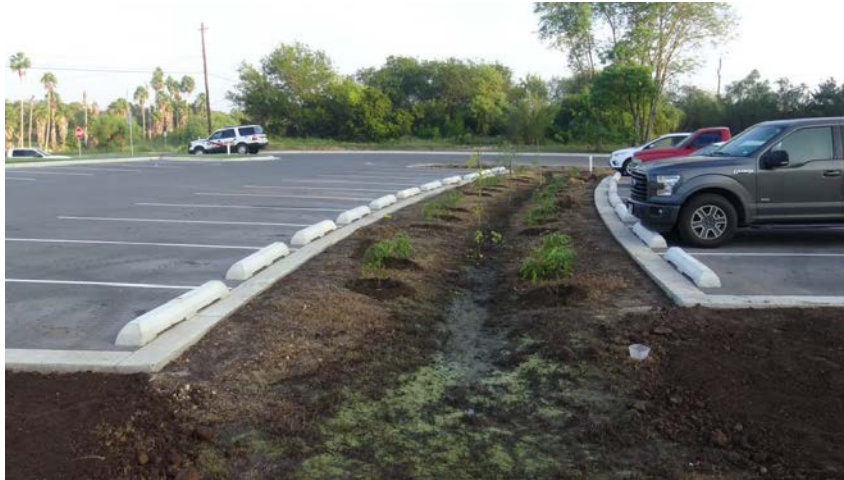
Native vegetation was recently planted in the Los Fresnos Nature Park bio-retention basin, looking from the south end of basin back toward the north.
