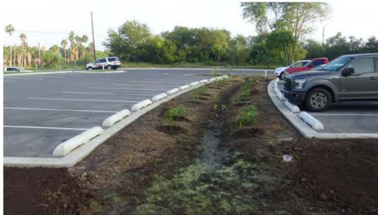
Native vegetation was recently planted in the Los Fresnos Nature Park Bio-retention Basin, looking from the south end of basin back toward the north.
