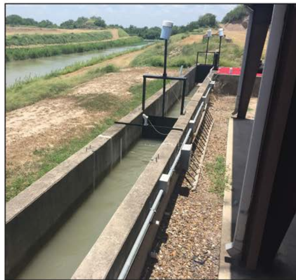
Water level sensor and automated gates in the demonstration channel at the Rio Grande Center for Ag Water Efficiency.
