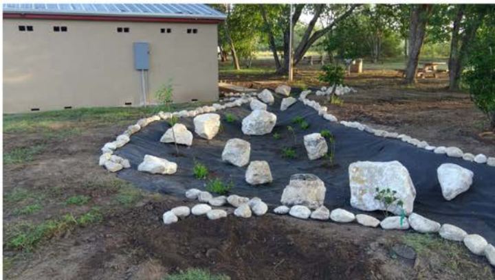
Vegetative swale and rain garden being installed and connected to the rainwater harvesting cistern to be installed behind the public restrooms.
