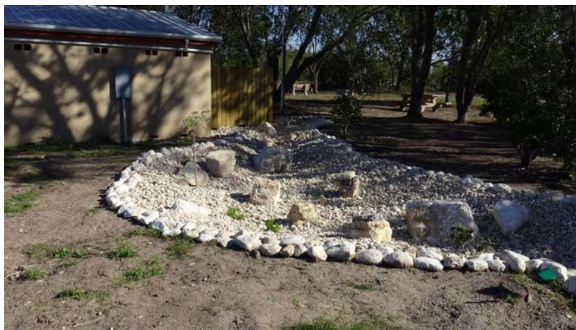
Swale with turk's cap planted in between boulders.
