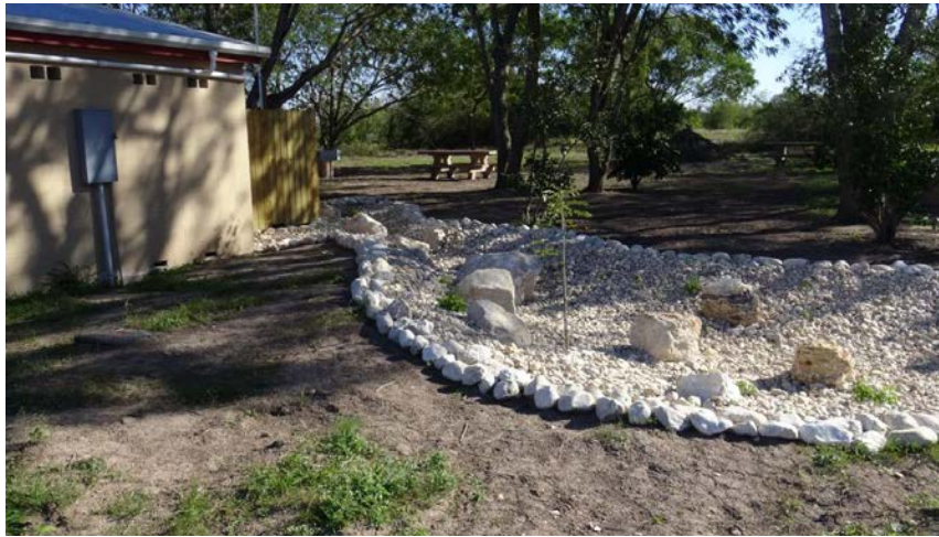
Completed landscaping on the vegetative swale and rain garden that is connected to the rainwater-harvesting cistern installed behind the public restrooms.
