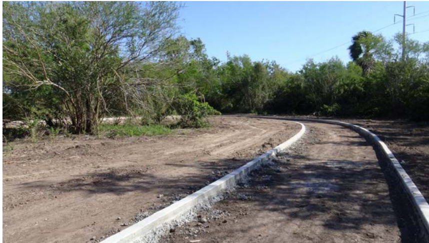
Heading north toward the U-turn. Concrete curb on both side of the trail is complete.
