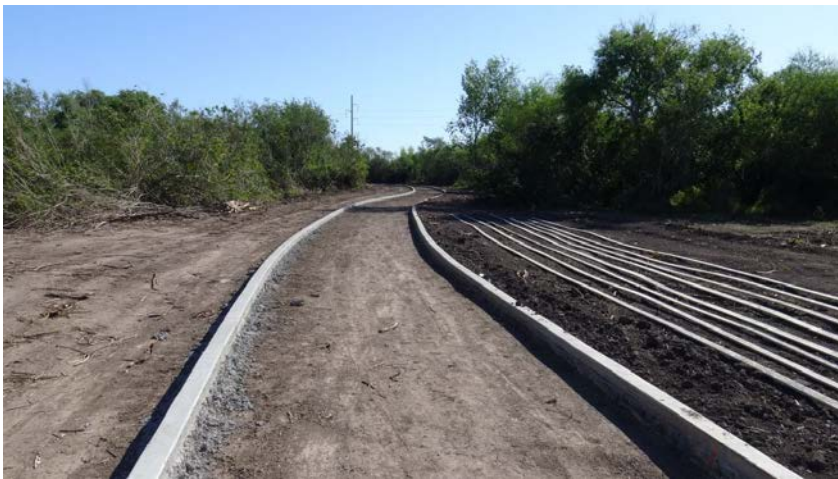
Heading east/northeast. The curb on the left side has been completed and the forms have been removed. The forms are visible on the right side of the photo.
