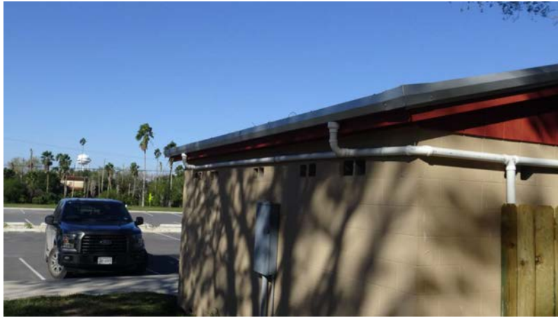
Plumbing of roof and rain gutters connecting to the rainwater harvesting collection system, southeast corner of bathroom looking northwest.
