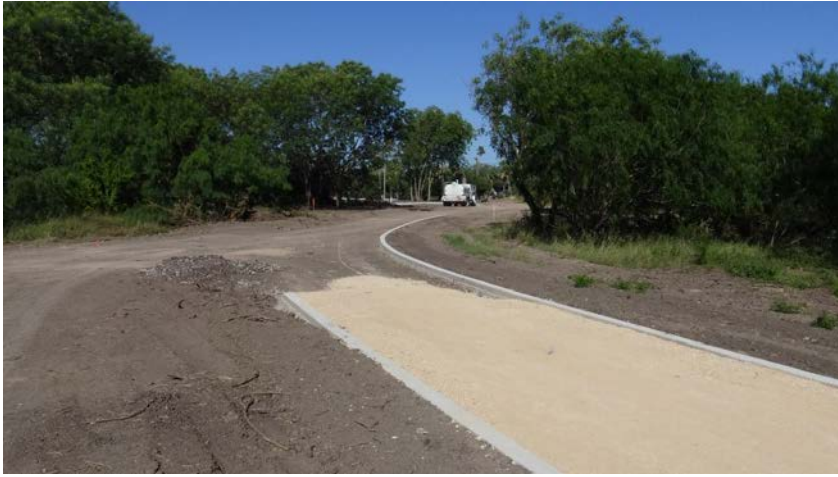
Heading north/northwest. This the last curb before the trail reaches the northeast side of the parking lot.
