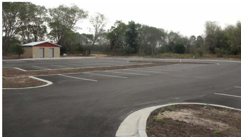
Looking SE and toward the bio-retention basin. Note the slope of the parking lot into the bio-retention basin.
