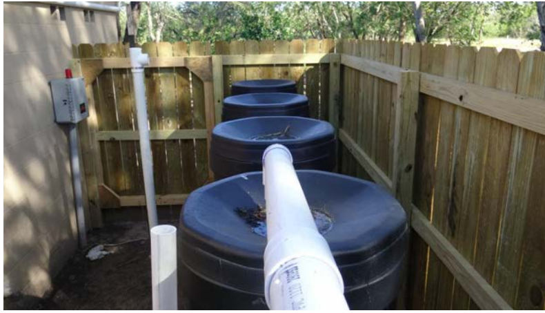
South view of the rainwater harvesting collection system connected to swale, south looking north.
