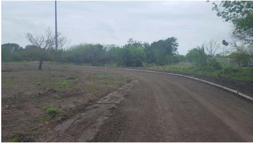
The high school tennis courts are visible on the right side of the picture. The form for the concrete curb that will define the edge of the walking trail is also visible.
