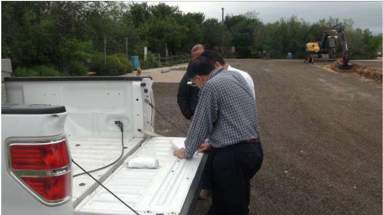
City of Harlingen Engineering Dept. checking specifications and verify elevations of the trench.
