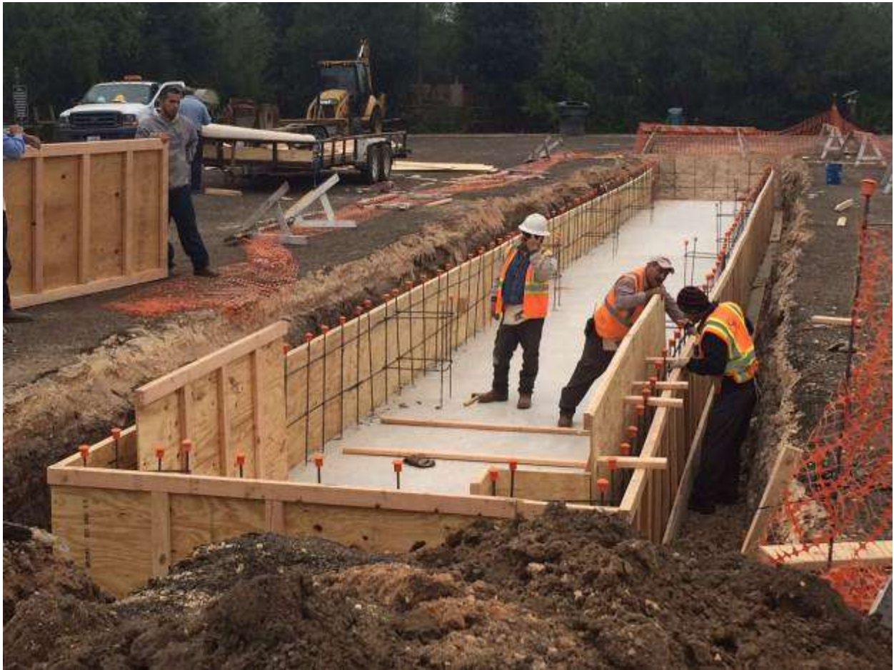
Once the concrete floor of the basin was poured and had time to set up, cure and dry properly, the COH began constructing the side walls of the basin.
