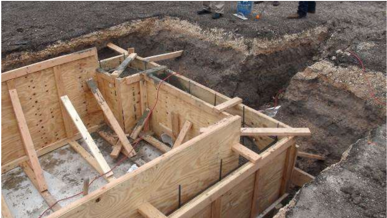
Installing the discharge pipe through the wall of the bio-retention basin that will drain the basin into the wetland system.
