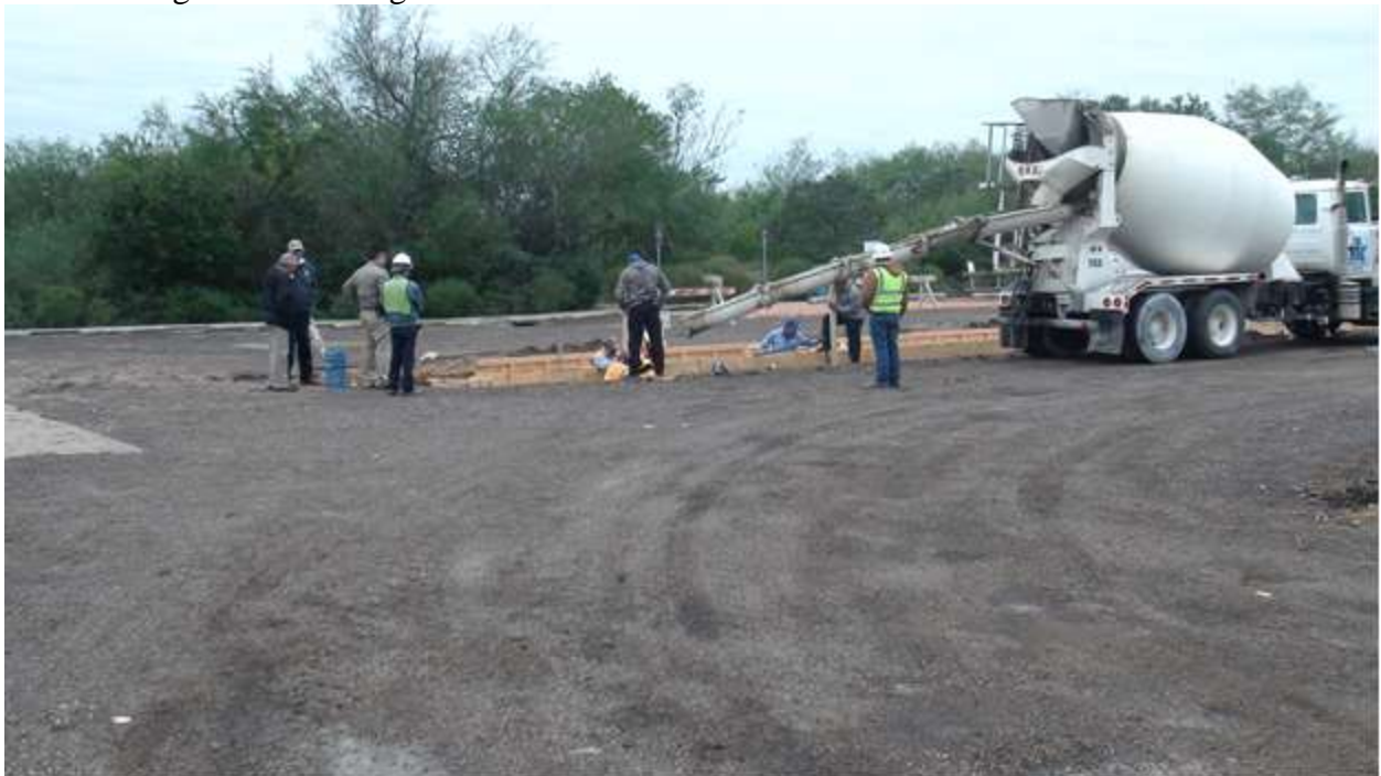
COH pouring the concrete for the side walls of the bio-retention basin
