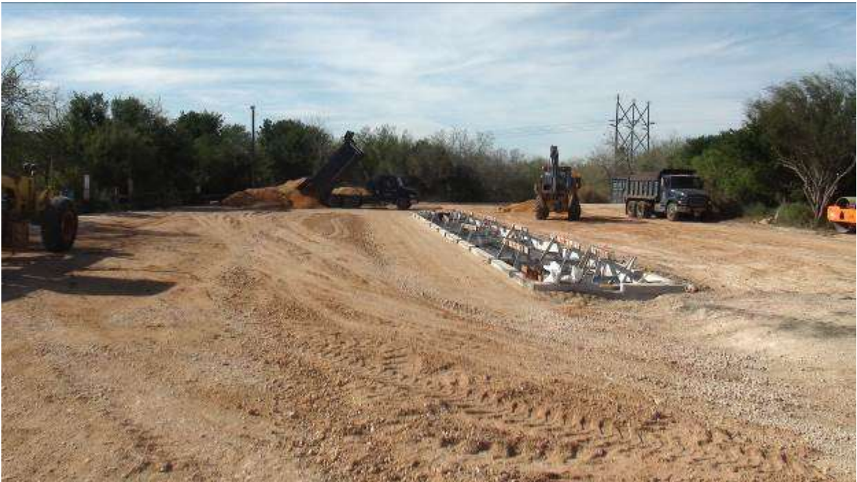
Cameron Co. crews installing new caliche in the parking lot in 1' lifts.
