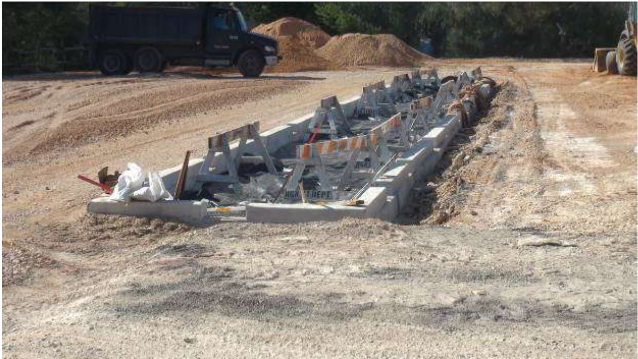
Preparing the slope in the parking lot to ensure that the storm-water drains into the bio-retention basin.
