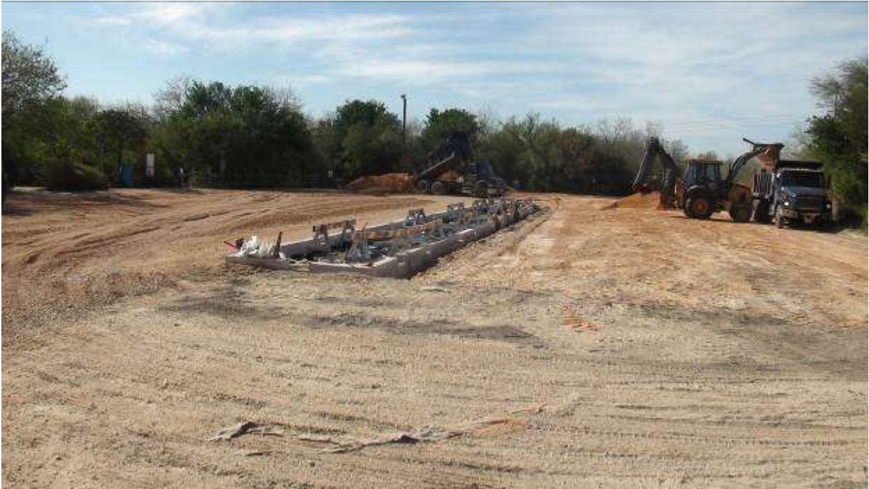
Cameron Co. crew removing existing sub-grade and caliche from the original parking lot.
